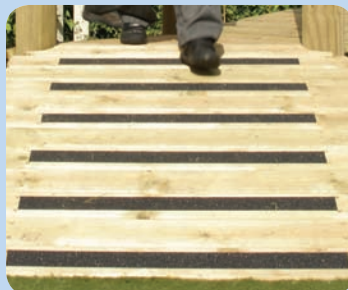
Anti slip strips on entry/exit ramps
